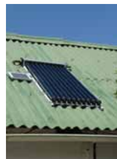
100L solar water heating system
